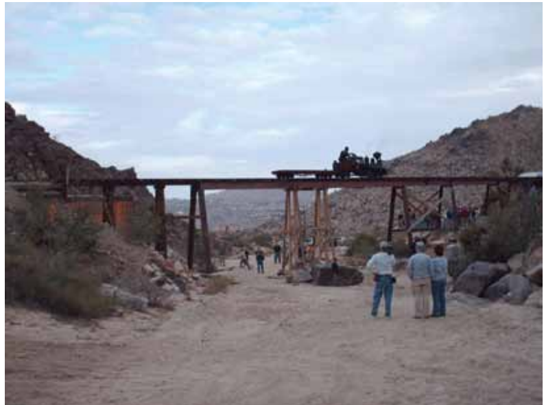
Quite a crowd has gathered to see a Grand Scale locomotive and flat car traverse the completed bridge armature over “Jack’s Gap” for the first time. The center pier has since been replaced with steel bents and a concrete footing, but the balance of the bridge structure has yet to be built.
