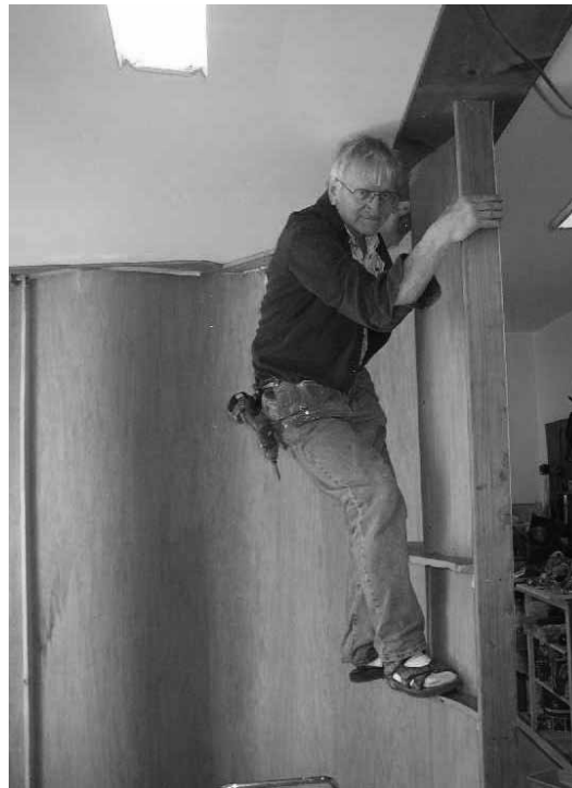
Walter Naumann shows that he's confident of the strength of Thin Wall construction by climbing on the first installed section. His feet are on the stiffening ribs set just below the layout's planned levels. Note also the wide boards screwed to the ceiling to provide convenient places to mount the upper anchor ribs. Two photos by Bruce Morden.
